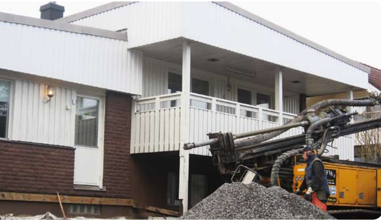
Drilling boreholes for a ground heat source heat pump for a typical house from the 1970s having waterborne electric heating.
