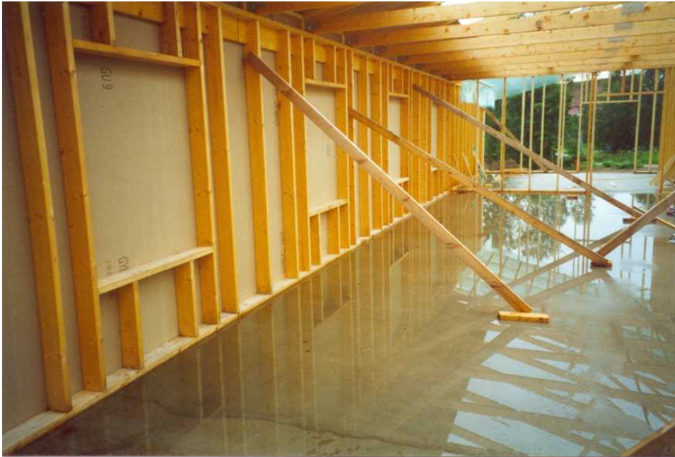
FIG. 2: An unprotected and wet building site with clear risk of future mould problems in the wooden structure, especially the sills. Photo: I Samuelson
